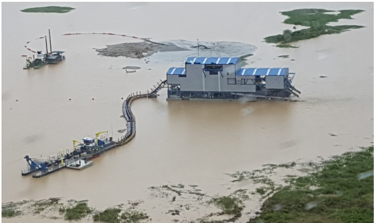
No. 20, No. 21 and Plant
